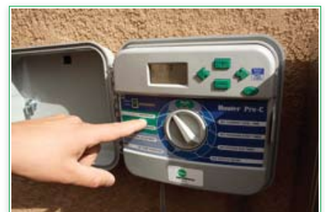
Sprinkler System Control, set to the OFF position.
